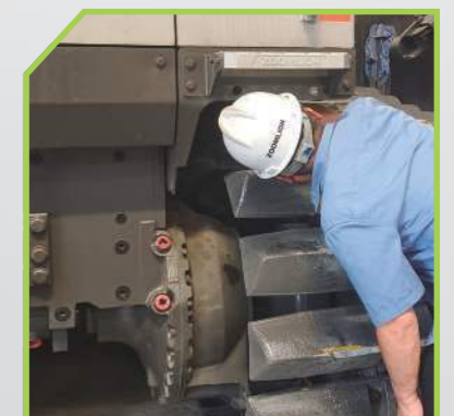
Oil tank draining 工作油箱放油
