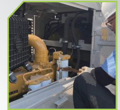
Fuel filter maintenance 燃油滤更换
