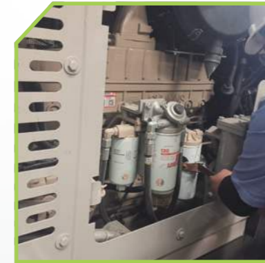
Oil filter maintenance 机油滤更换
